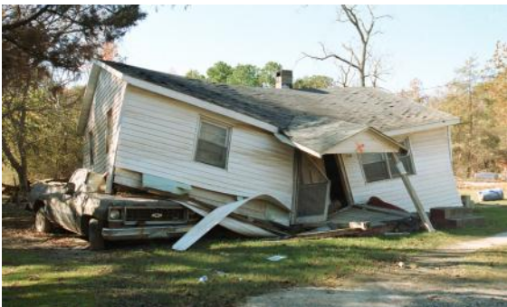
The roof and walls of this home have been compromised and it is off its foundation.
