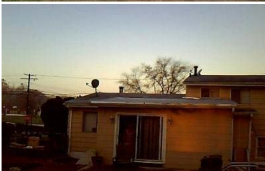
The roof on this residence has been tarp covered after it lost some shingles.
