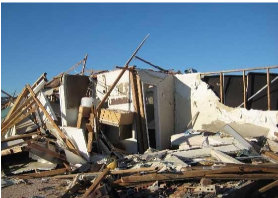
This residence has collapsed.
